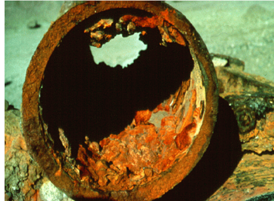
Salinity damages to municipal water pipe.
